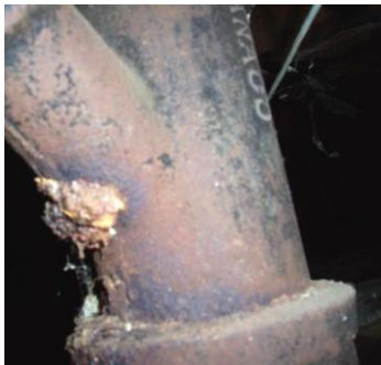
1. Pinhole leak in a cast iron drain pipe.
