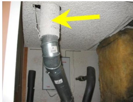
Figure 2. Possible asbestos insulation on water heater exhaust flue.
