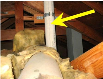
Figure 1. Possible asbestos insulation on furnace exhaust flue in attic.
